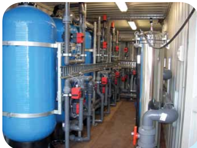
Sea water pre-filtration unit for Chevron's Gorgon LNG project
