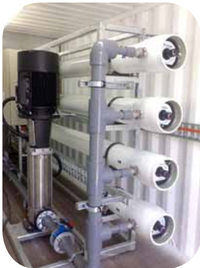
Reverse Osmosis Plant (1,000m 3 /day) for bore or CSG water treatment
