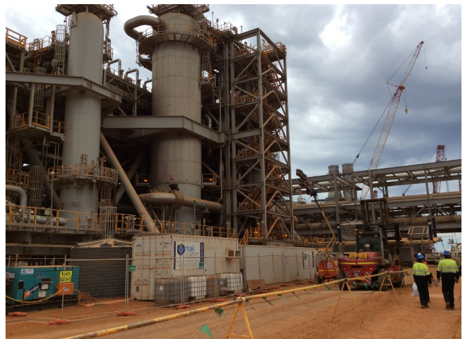
The two Brackish Water Reverse Osmosis hire plants were customised and delivered within four weeks
