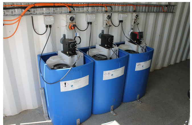
Chemical dosing systems
