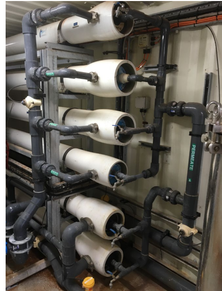
Reverse Osmosis vessels
