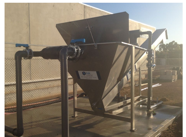
Innovative sludge removal system installed on site in Bunbury
