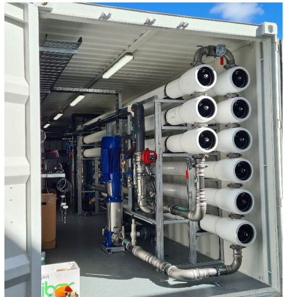
MAK Water BWRO hire plant in testing bay at MAK Water factory
