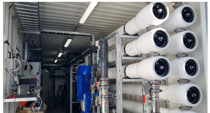
Internal view of the BWRO hire plant
