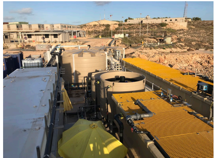
View across the sewage treatment facility
