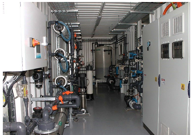
Internal view of the containerised BWRO plant
