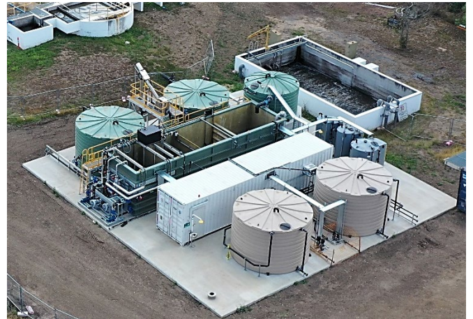
Aerial view of the MBR and BWRO installation
