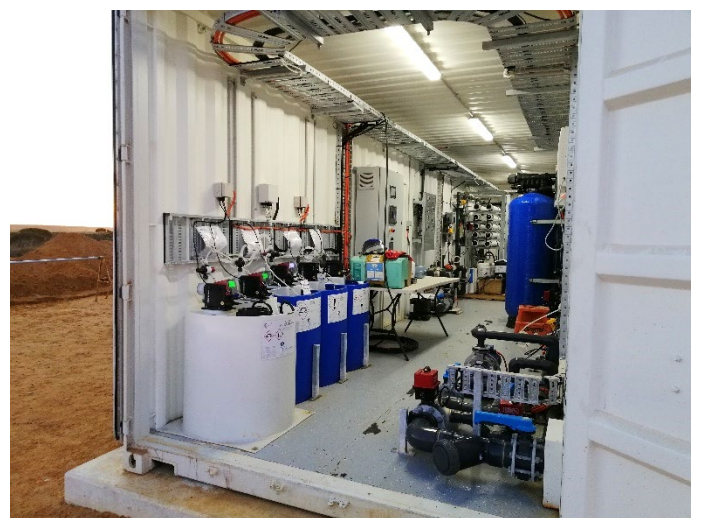
Internal view of the containerised SWRO plant
