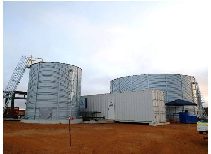
MAK Water containerised SWRO plant installed onsite
