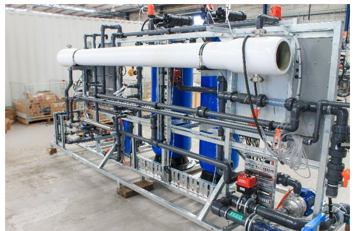
RO vessel on rear of skid
