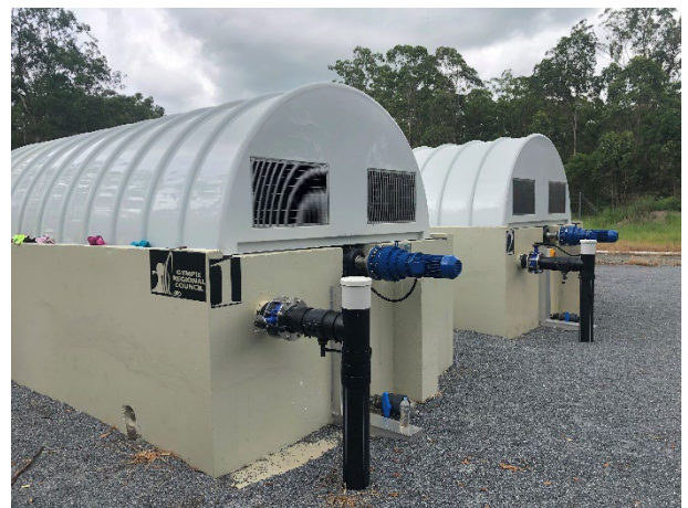
Rotating Biological Contactors
