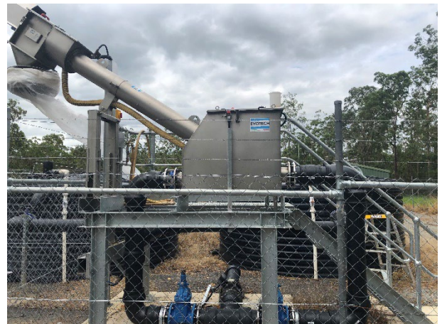
Screw Screen in Tank
