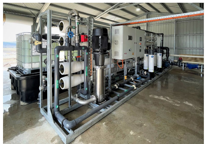
BWRO installed at piggery in Queensland
