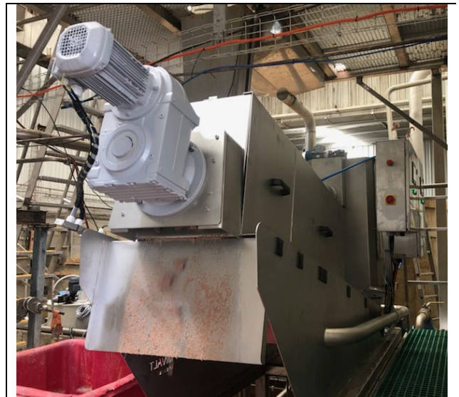
Commissioned Dewatering Screw Press with Raised Platform
