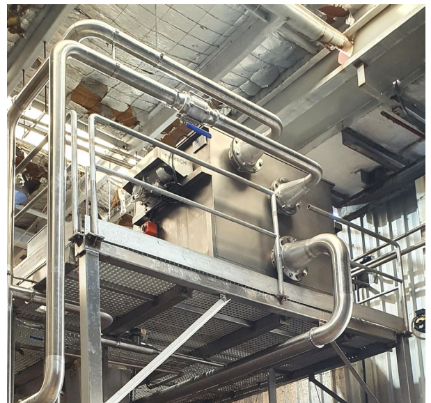
Commissioned Rotary Drum Screen (FTR) with Screw Compactor (SCC)
