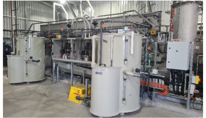
DAF system with Polymer Preparation Systems (ASPs) in foreground
