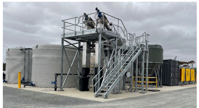
Left to right; Balance tanks, Influent Screens on custom elevated platform, Sludge Tank, 40' containerised plant room, self-bunded chemical storage & dosing cabinets.
