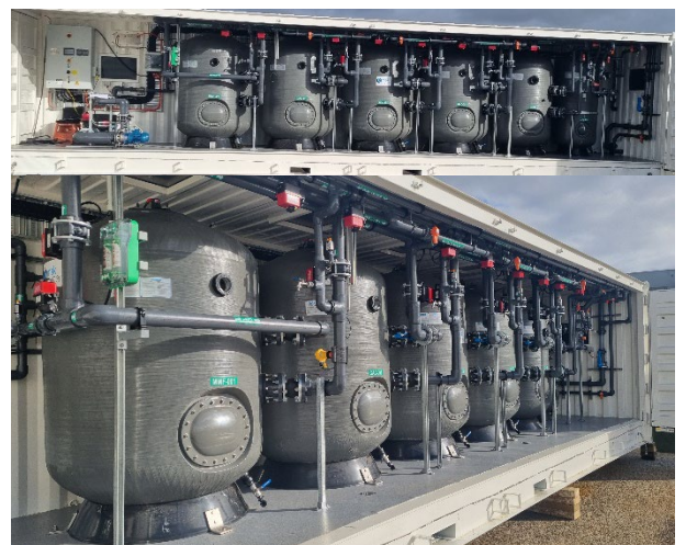
Two photos of one of the filtration plants in the testing bay at the MAK Water factory
