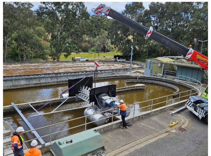
One of the Floating Brush Aerators being installed in an oxidation ditch. This solution can be quickly installed and uninstalled to meet peak demand seasons
