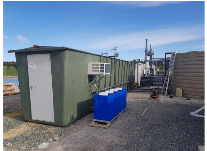
MAK Water ASBR hire plant installed onsite
