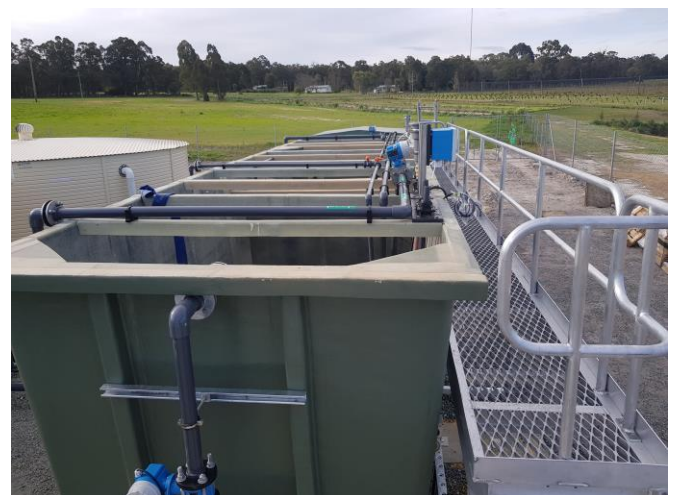
MAK Water ASBR hire plant with access platform
