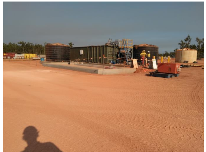
MAK Water ASBR plant onsite in North Queensland
