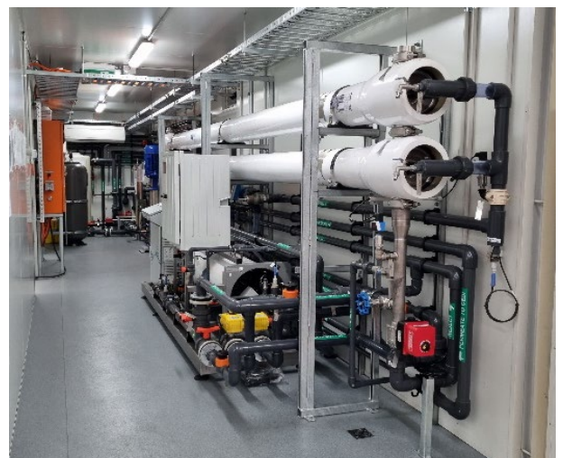
Reverse Osmosis and Continuous Electrodeionisation plant
