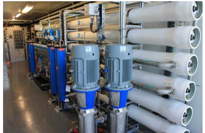
Demineralised Water Treatment Plant (BWRO + CEDI)
