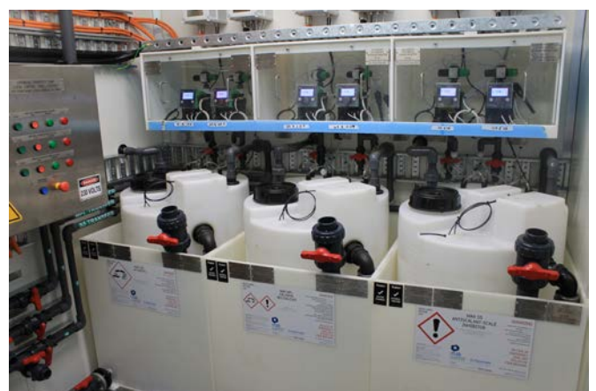
pH Correction and Dosing system
