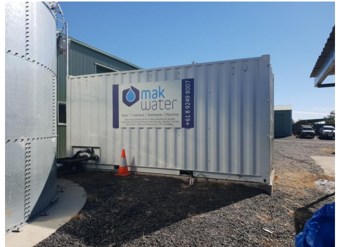
Brackish Water Reverse Osmosis (BWRO) Plant on-site in Queensland
