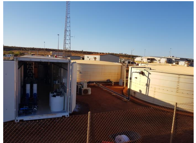
Containerised Brackish Water Reverse Osmosis plant installed onsite
