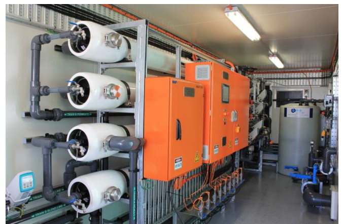
BWRO plant during FAT at MAK Water's Perth manufacturing facility
