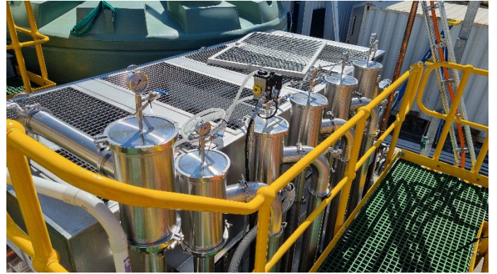
Above- view of the GEM-DAF component, showing one of the removable cover grid sections,
