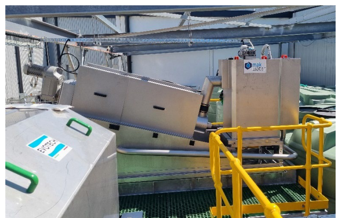
Rotary Drum Screen (FTR) left, Dewatering Screw Press (DSP), centre.
