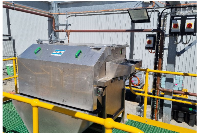
Influent solids screening - Rotary Drum Screen (FTR) installed on elevated platform. Screenings drop into a bin below the elevated deck.
