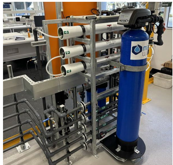
RO Vessels and Multimedia Vessel with advanced control valve head.
