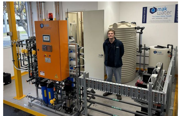
MAK Water BWRO plant installed at North Metro TAFE
