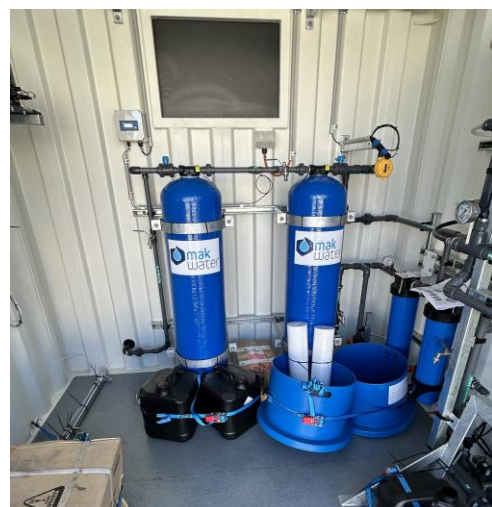
Brackish Water Reverse Osmosis (BWRO-B-010)
