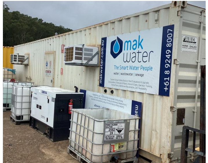
Brackish Water Reverse Osmosis (BWRO) plant
