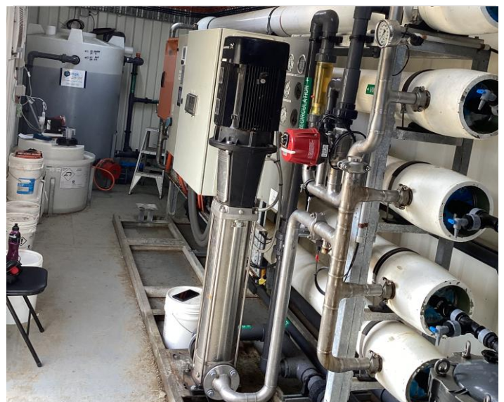
Sea Water Reverse Osmosis (SWRO) plant
