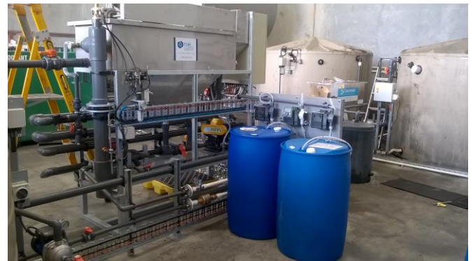
MAK Water OWS, Flocculation and DAF system in workshop
