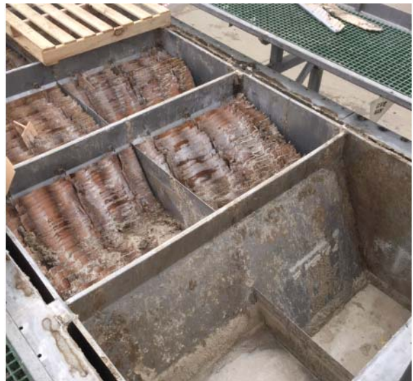
Collapsed and damaged plate packs in DAF
