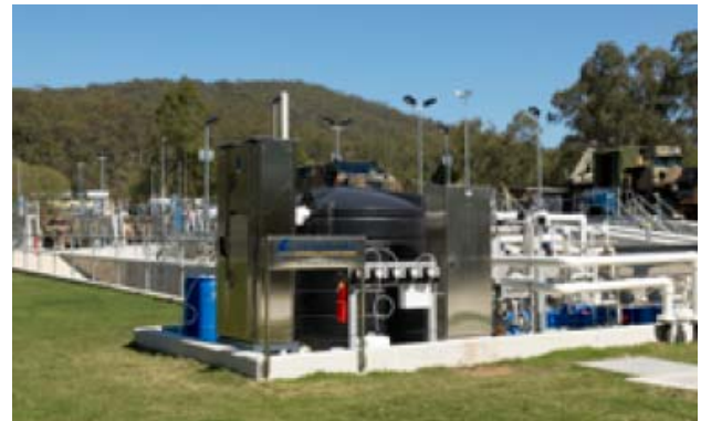
The dissolved air flotation wash bay water recycling system on site at the Enoggera Barracks
