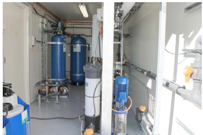
Containerised Brackish Water Reverse Osmosis Plant
