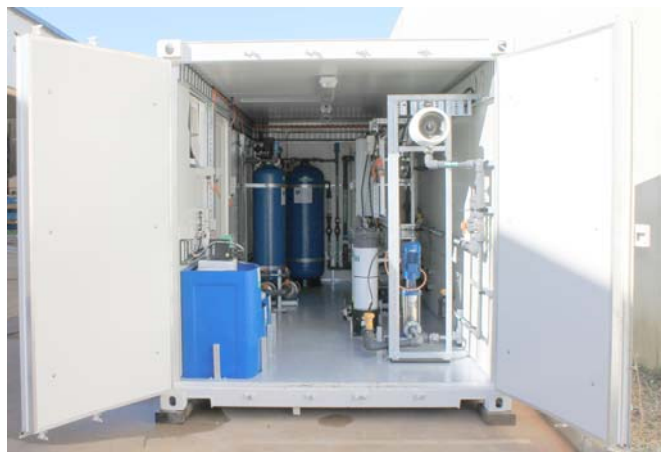
Containerised Brackish Water Reverse Osmosis Plant
