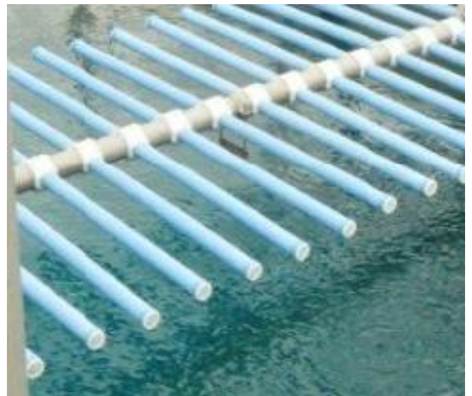
In tank aeration diffusers
