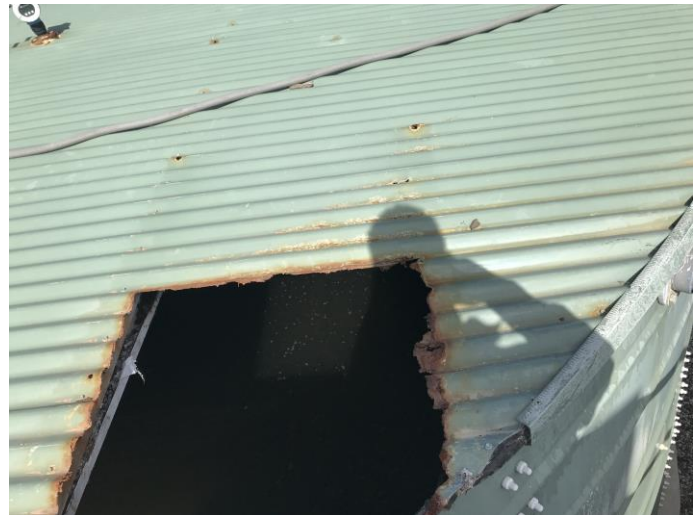
The existing roofs had extensive damage
