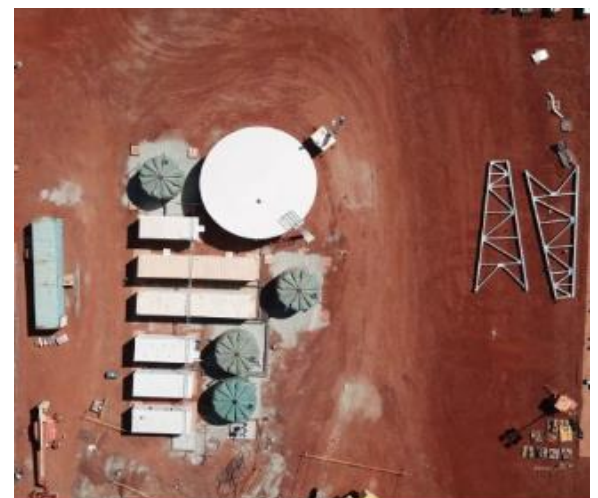
Arial view of MAK Water installation on site
