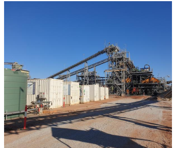
MAK containerised water treatment plants on site
