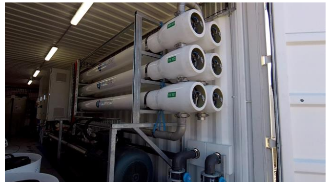
Containerised SWRO plant
