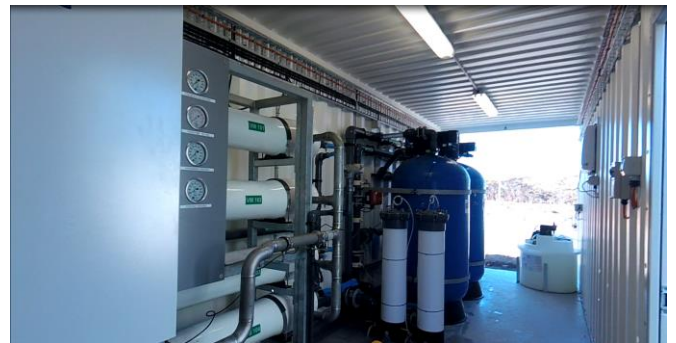
Containerised plants onsite
