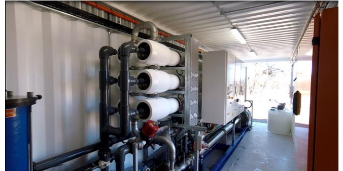
SWRO plant installed onsite
