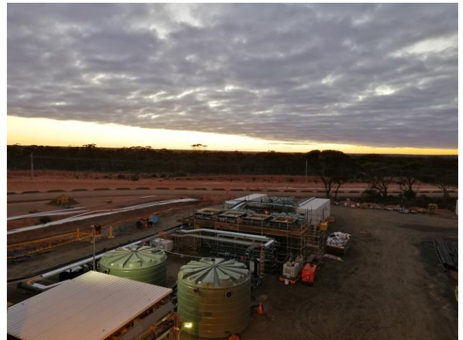
SWRO and LC plant installed onsite
