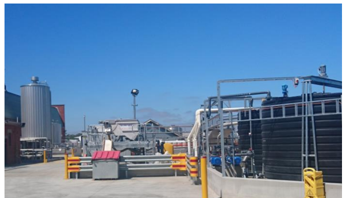
Salsnes Fine Screen Filter and pH correction system on site
