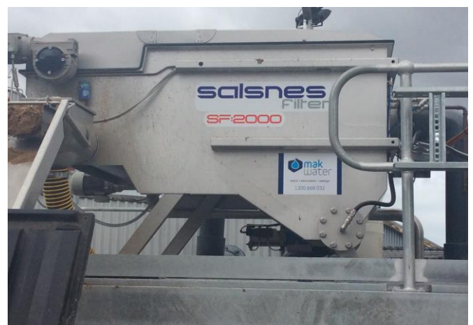
MAK Water provided all site installation works and commissioning as part of the turnkey solution
