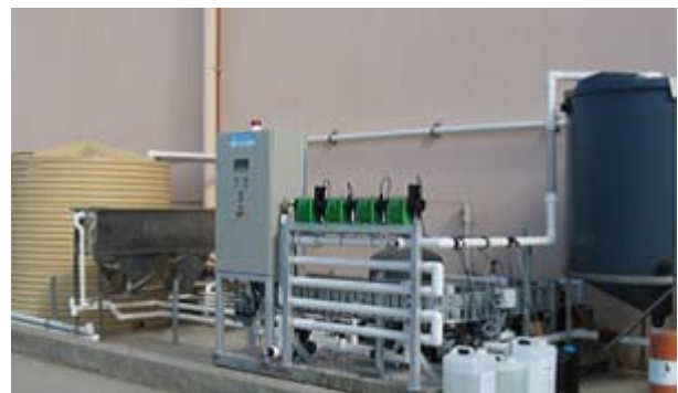
Upgraded wash down recycling system operates at current best practise efficiency
