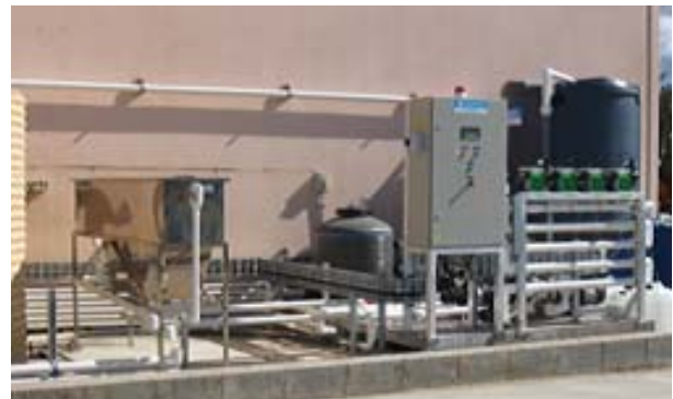
Peachey Constructions' upgraded wash down recycling system
