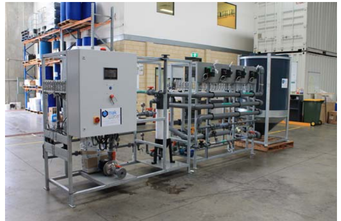
The completed gravity clarification system in the MAK Water workshop
