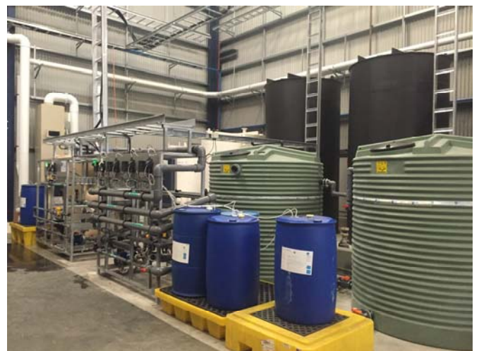
The gravity clarification system installed on site at SuperCharge Batteries.
