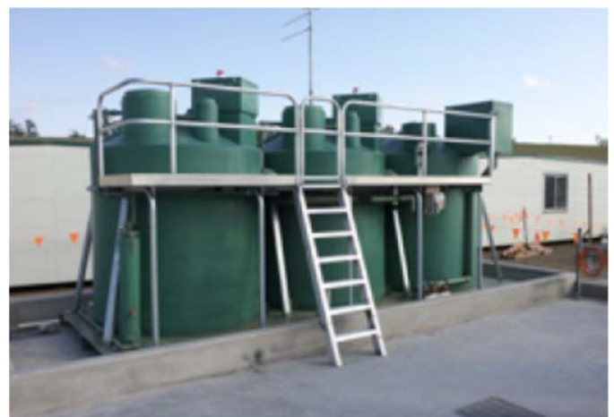
Custom engineered aerobic primary treatment process and sterilisation
