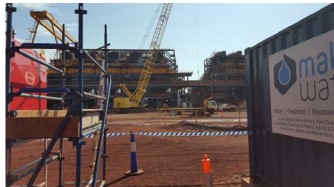
The sewage treatment plant on site in the Pilbara
