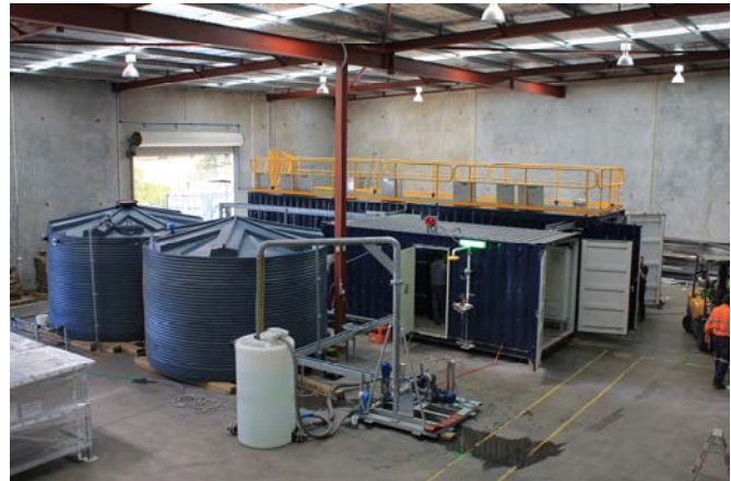
Moving Bed Bioreactor Sewage Treatment Plant
