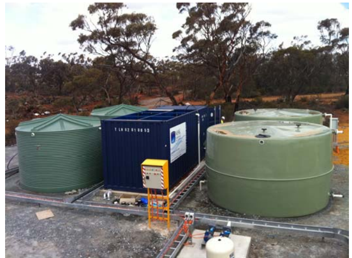
Membrane Bioreactor Sewage Treatment Plant installed on site
