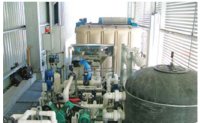
Water efficient wash bay
