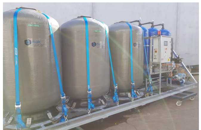
Multimedia Filtration Plant for PFAS removal on it's way to site
