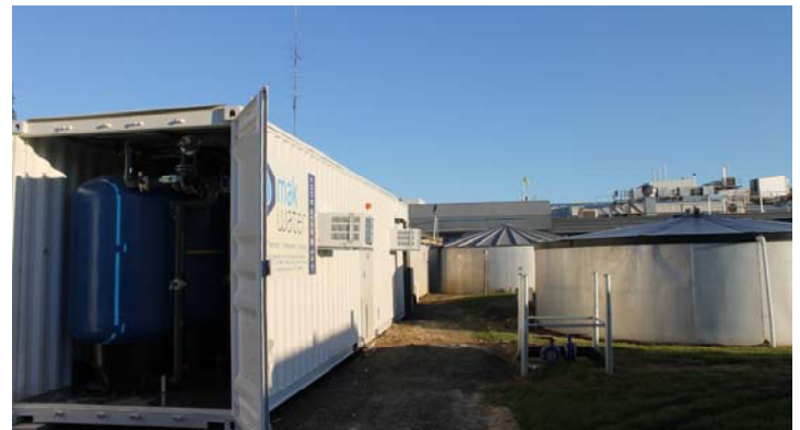
MAK Water containerised MMF plant installed onsite
