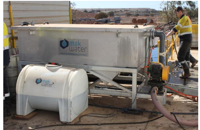
CL10 Oil Water Separator installed onsite
