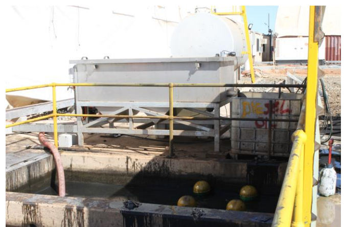
Floating Suction Skimmer and OWS system
