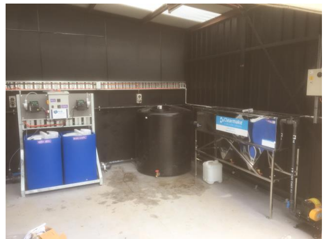
PAF and OWS installed onsite
