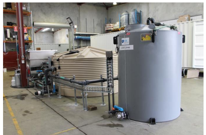
2,300L self-bunded waste oil storage tank
