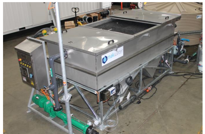
Separator skid with feed pump, control panel and overhead lighting tower
