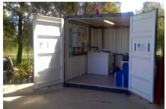
pH Adjustment Batch System capable of treating up to 1,000l/h of acid wastewater
