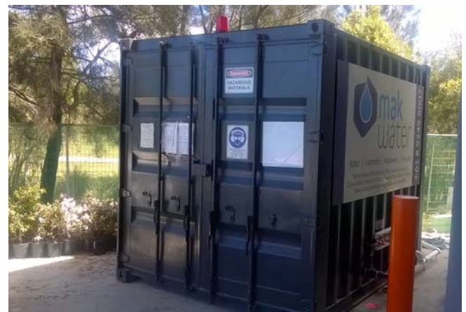
Containerised pH Adjustment Plant
