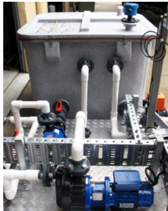
pH Adjustment Plant
