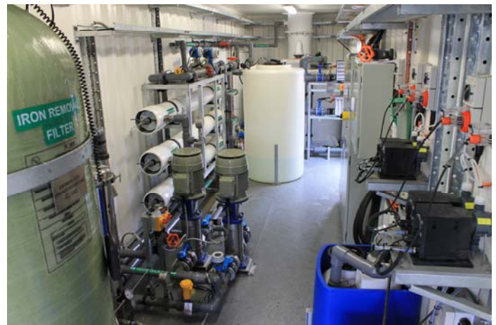
Containerised demineralised plant
