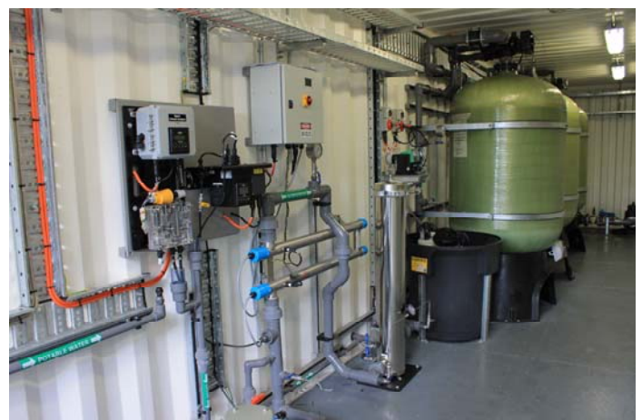
Potable water treatment plant
